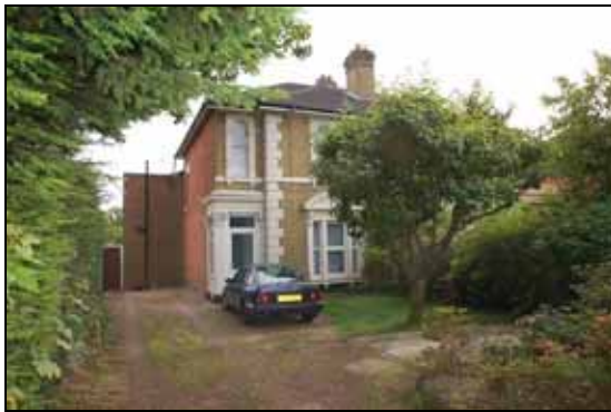
74 Portsmouth Road – The porch has been enclosed with upvc units and the original windows have been replaced with upvc.
