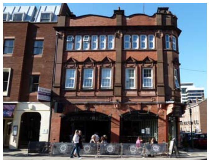
Good detailing undermined by the use of uPVC windows, 31 and 32 Oxford Street
