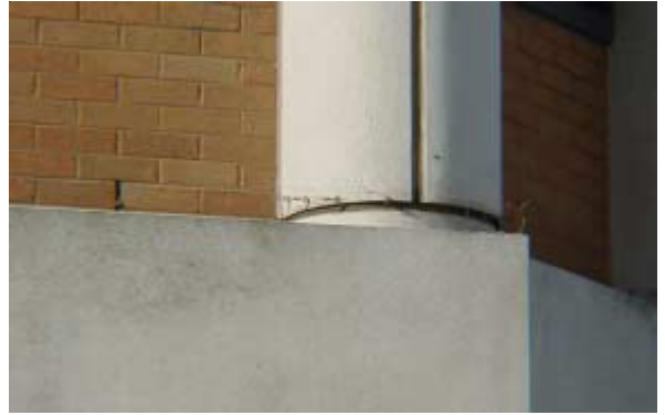
Use of wires and spikes fixed over ledges will prevent birds from perching.
