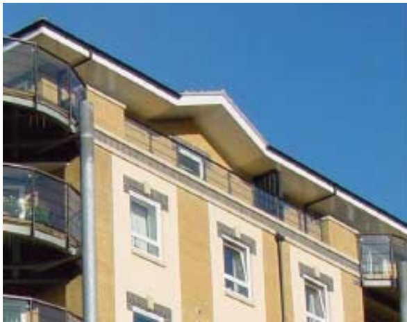
This roof plane is not sufficiently dominant; the white fascia boarding is inappropriate for an urban location.
