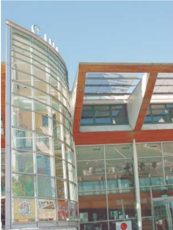
Roof detailing of the Harbour Lights Cinema has resulted in differential weathering of the timber finishing, marring an otherwise exquisite façade.
