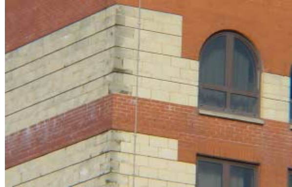
Poor quality concrete facing blocks show the effects of porosity in an exposed location.
