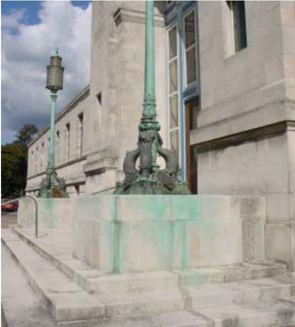
Copper oxide stains on plinth.
