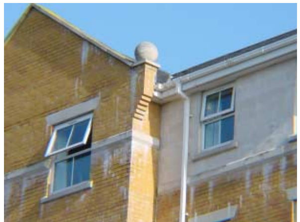
Sulphates leach out of the concrete details causing severe staining.
