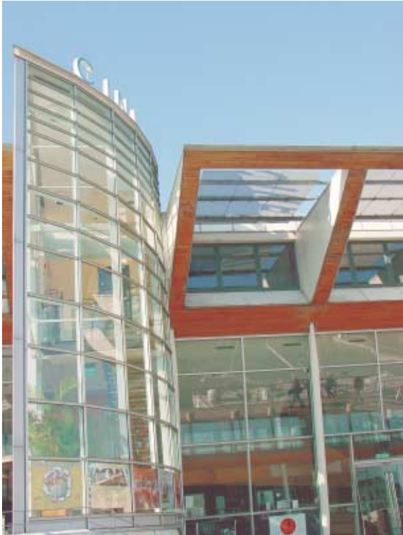
Roof detailing of the Harbour Lights Cinema has resulted in differential weathering of the timber finishing, marring an otherwise exquisite façade.
