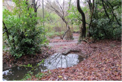
Photo 6: Blocked piped section under a footpath
