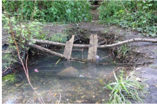
Photo 3: Area with suspected damaged surface water sewer
