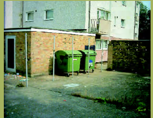
Waste storage areas should be provided to prevent eye-sores such as this
