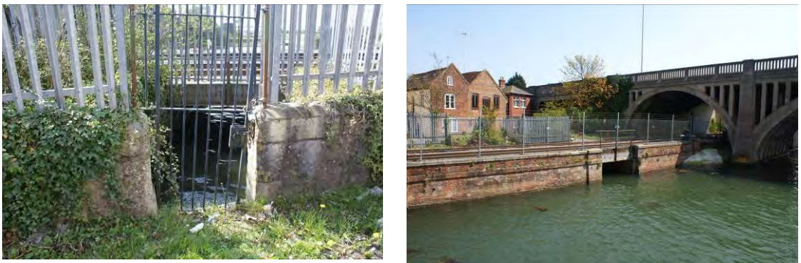
Figure 6-17. Photographs of the gap in the wall near the Redbridge road bridge.
