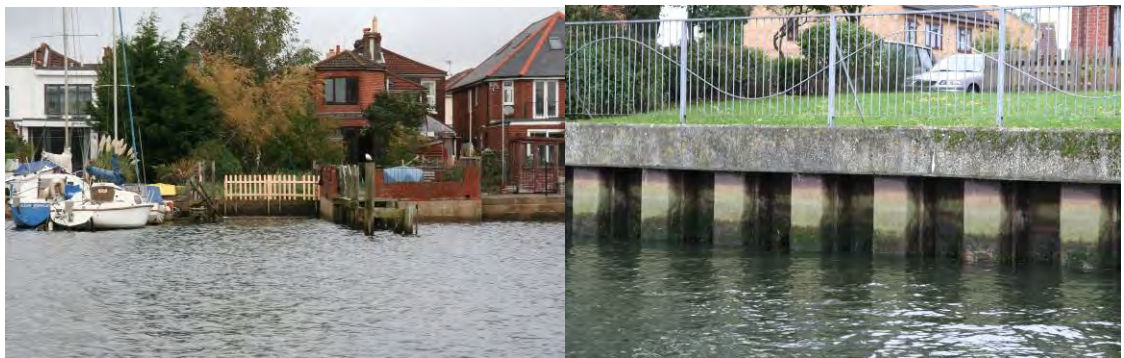
Figure 5-1. Informal private defences on the Upper Itchen (left) and formal steel sheet pile erosion defences (right).
