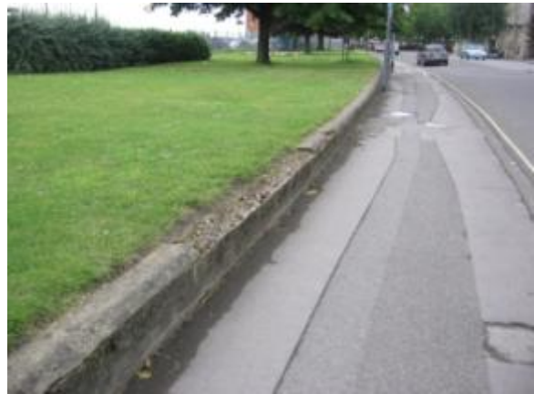
Figure 50. Poor asphalt paving and kerb,
