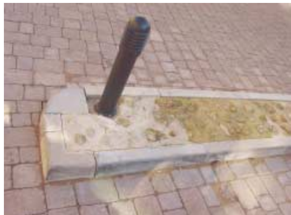
Attention to detail is crucial; this raised area in a car park is very poorly finished. The cobbles are spaced too far apart, giving emphasis to the mortar filling which has been laid in two batches of different mixtures. The bollard is too close to the kerb to allow cobbles between it and the kerb.
