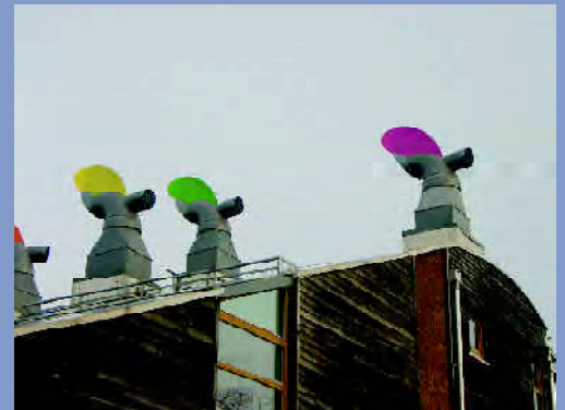
Ventilation cowls are designed as an integral feature of this sustainable development - BedZed
