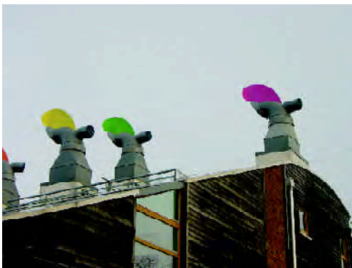
Ventilation cowls draw out hot air providing natural ventilation by the 'stack' effect - BedZed
